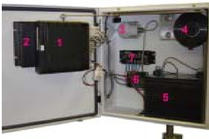
Inside the Extensometer Enclosure
